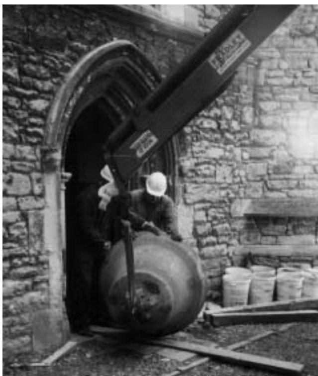
Removal of the tenor bell required partial dismantling of the west door
